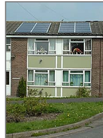
Figure 3: Example of Retrofitted Solar Panels
